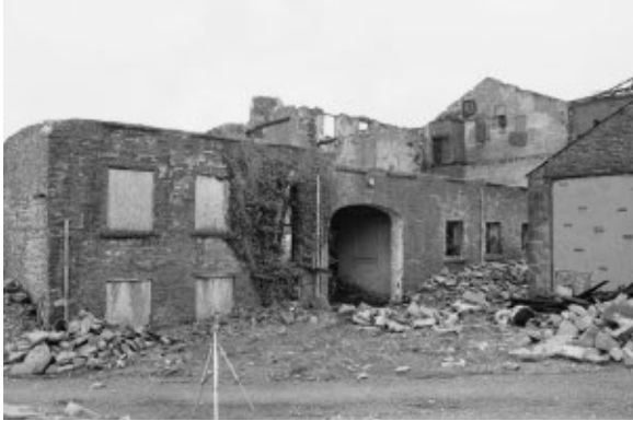
View of the north side of the badly damaged rear three storey building with the boiler house on the right.
