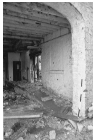
View from the north side of the archway under the rear three storey building.
