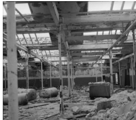
Looking south in the weaving shed with the intermediate wall on the right.
