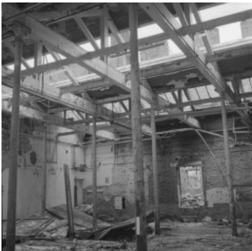
Looking north at the south wall of the rear three storey building from the 1907 extension.
