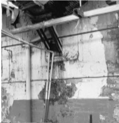
Bearing box, on centre line of columns, in eastern end wall of the weaving shed.
