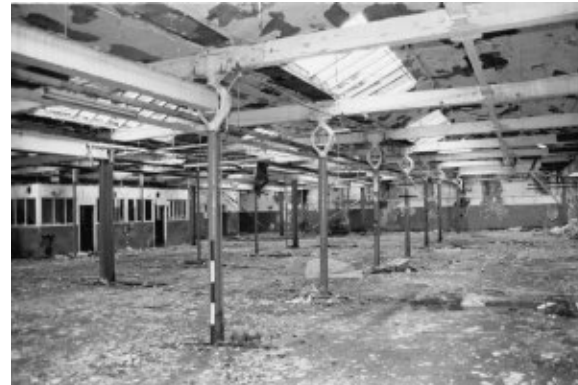
View looking eastwards from the central dividing wall in the weaving shed looking towards the wall behind which the steam engine was located.
