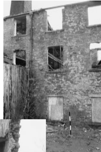
North facing wall of the front three storey building with the down spout hopper dated 1839 on the left.
