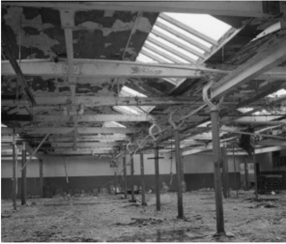
Looking west from the east wall of the weaving shed showing the central line of columns with bearing housing for the drive shaft.
