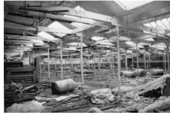
View across the weaving shed from the south east corner showing old fixings for bearing supports rebated centrally into the roof support beams.
