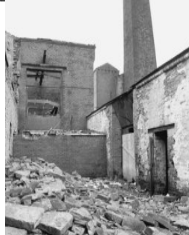
Looking west at the brick extension to the engine house with the boiler house on the right.
