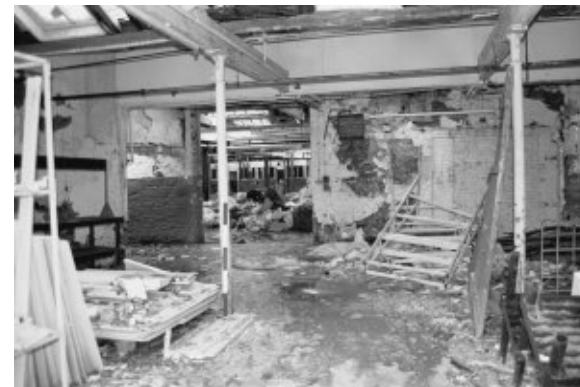
Looking north into the weaving shed from the entrance to the southern single storey extension.
