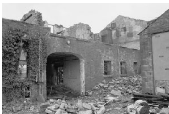
View of the north side of the badly damaged rear three storey building with the boiler house on the right.
