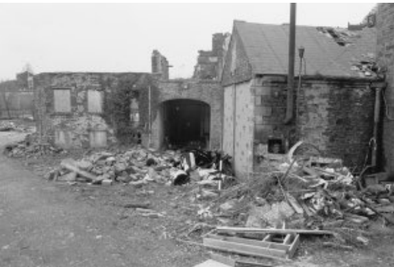
Looking south at the north wall of the rear three storey building with the boiler house on the right.
