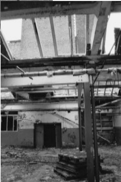
View looking to the north at eastern end of the weaving shed showing the lift shaft built outside of the front three storey building and the location of the chimney.
