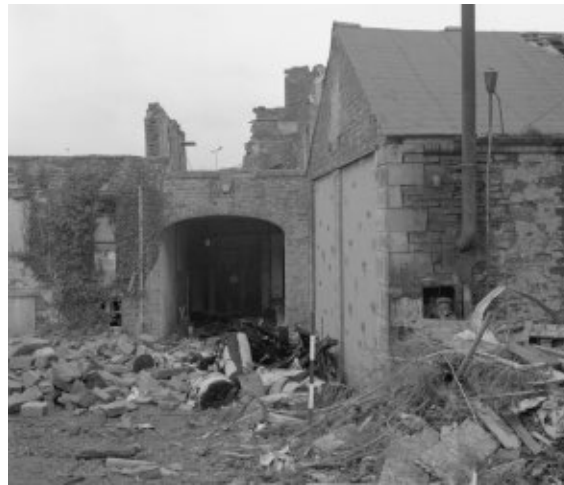
Looking south at the archway under the rear three storey building with the boiler house on the right.
