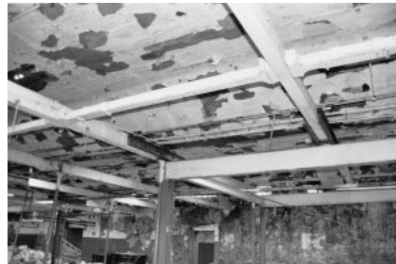
Cast iron carriers for the transverse line shafting fitted between the beams supporting the roof. Additional steel RSJs have also been installed to allow one line of cast iron columns to be removed.
