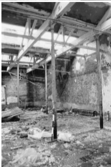
Inside of 1907 extension looking northwards to wall of rear three storey building and showing an infilled window on the left.
