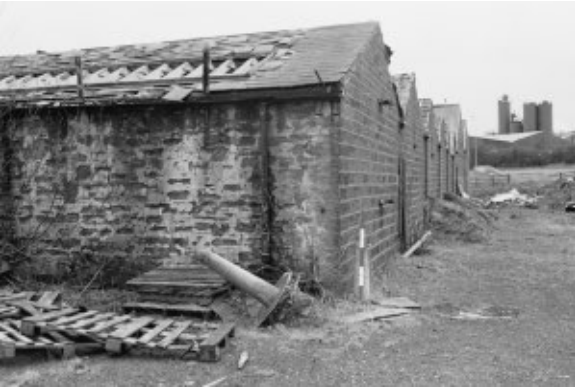
Looking south along the west face of the weaving shed showing the water-shot stone-work.
