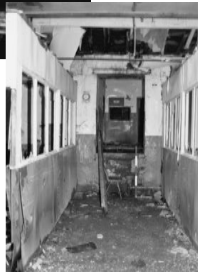
Looking north at the south wall of the front three storey building from the weaving shed.
