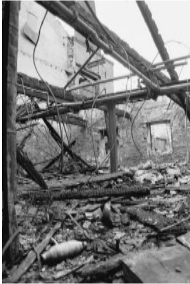
Looking north west inside the remains of the rear three storey building at the intermediate wall, behind which was the engine, from the 1907 extension.
