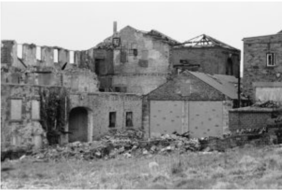
Looking south west at the north face of the rear three storey building and the boiler house.
