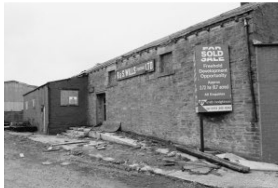
View along the south wall of the 1907 extension with date stones next to the doorway.
