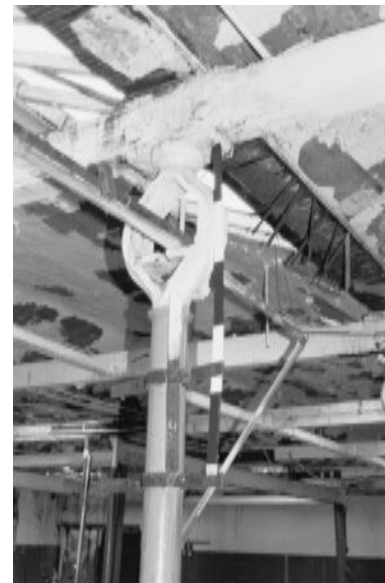
Typical bearing housing in top of cast iron columns in the weaving shed.
