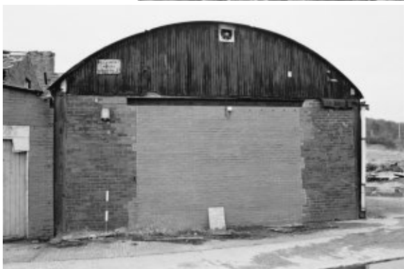
South face of metal framed building at the south east corner of the collection of buildings.
