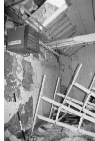
North east corner of the single storey extension on the south side of the weaving shed showing the angled wall which was part of the 1907 mill extension and the brick filled former doorway.
